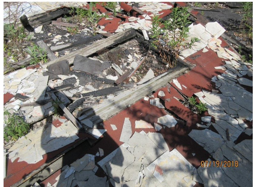
Photo 12 – Broken Transite debris on the southeast portion of the site
