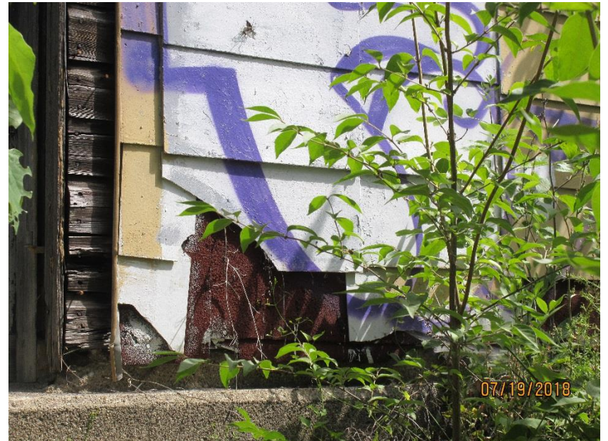
Photo 14 – Broken Transite siding on the southwest building on the site
