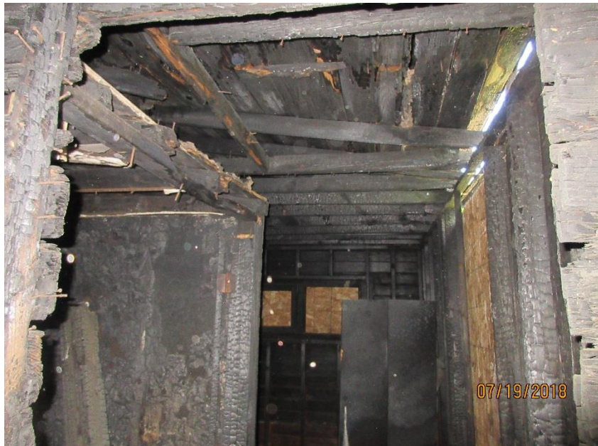
Photo 7 – Fire damage to the building frame of the southwest building on the site
