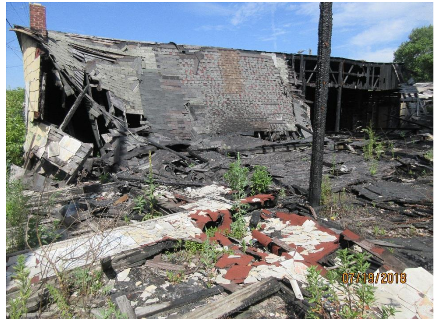
Photo 8 – View showing collapsed roof on east side of the southwest building and debris across the site
