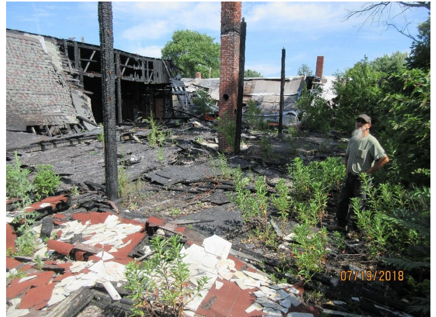
Photo 10 – View of debris covering the site as seen looking to the northwest
