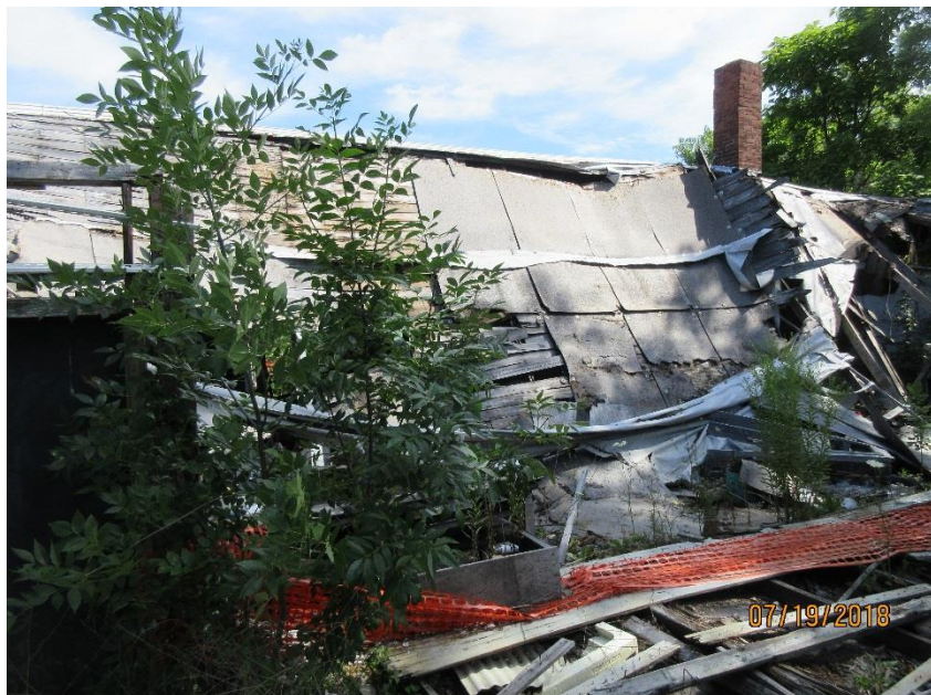
Photo 11 – View showing collapsed roof over the south wall of the north building on the site
